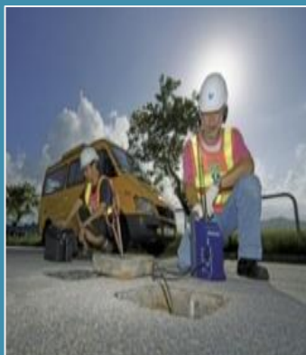
Active Leakage Detection & Control
