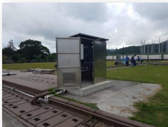
Water Quality Monitoring Station
